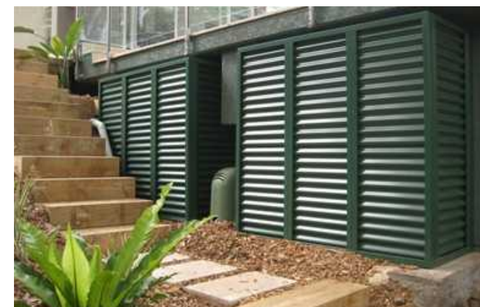
Figure 34: An example of concealed tanks used for rainwater harvesting
