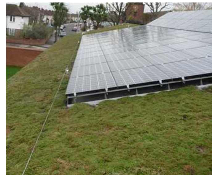
Figure 35: Green roof combined with solar panels.
